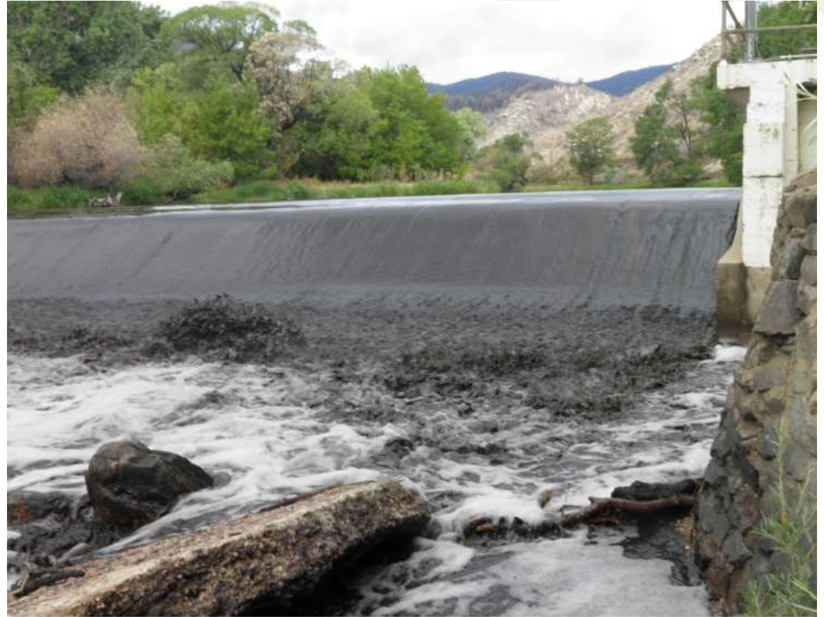
Greeley's Bellvue Treatment Plant Diversion Dam following post fire precipitation and flood event
